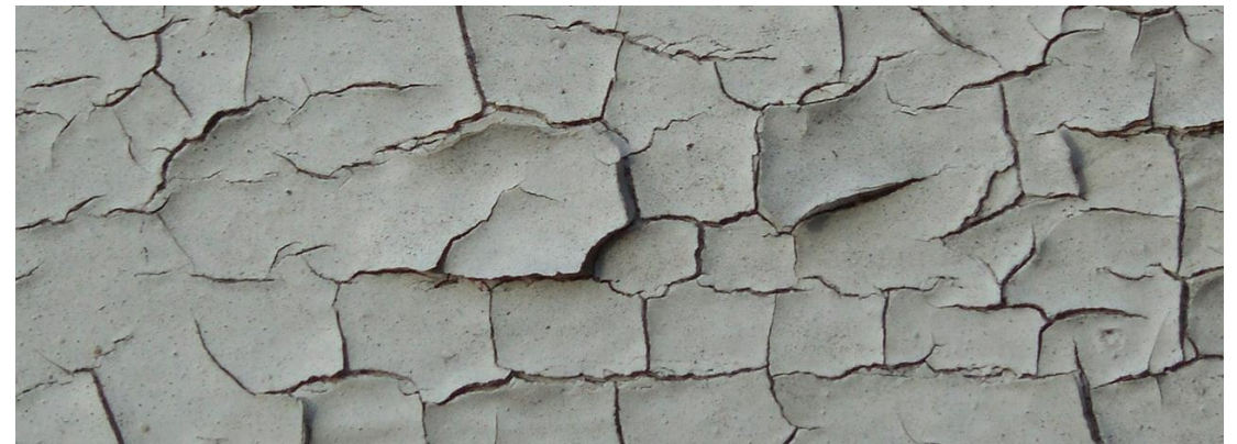
Leaded paint can be identified by this “alligatoring” flaking pattern
